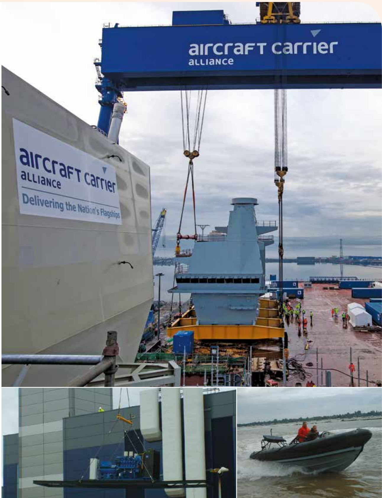
TOP: The Aft Island of the latest QEC Class Aircraft Carrier, HMS Prince of Wales, is carefully lowered into position ready for Tex "Flyco" installation.
